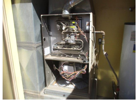
Heating 1st Floor Rear:
