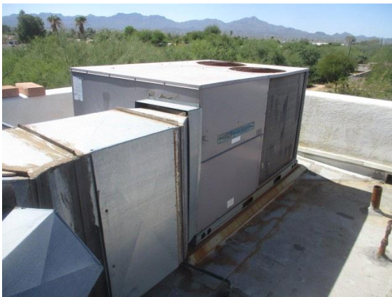
Heating 1st Floor West:
