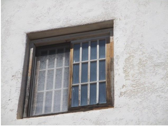
Windows: Needs Paint
