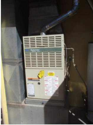
Heating 1st Floor Rear:
