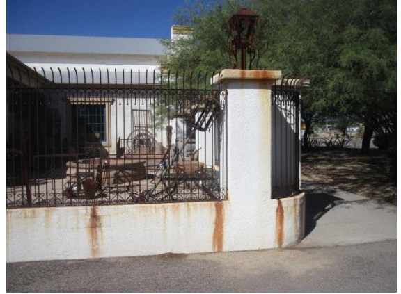
Fences / Enclosures: Rust Stains
