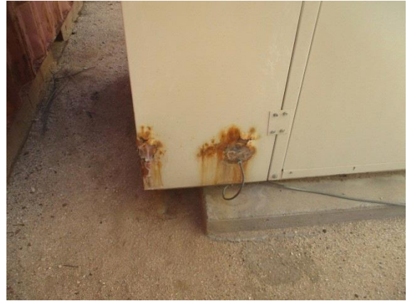
Cooling 1st Floor Rear:
