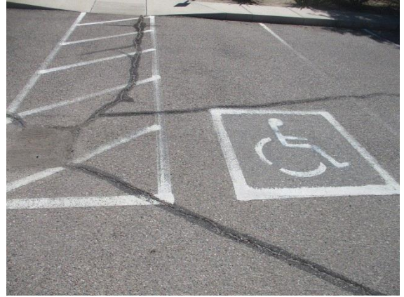
Parking Lot / Driveways: Parking Stripes Faded
