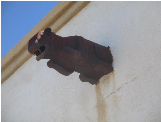
Roof Drainage System:
