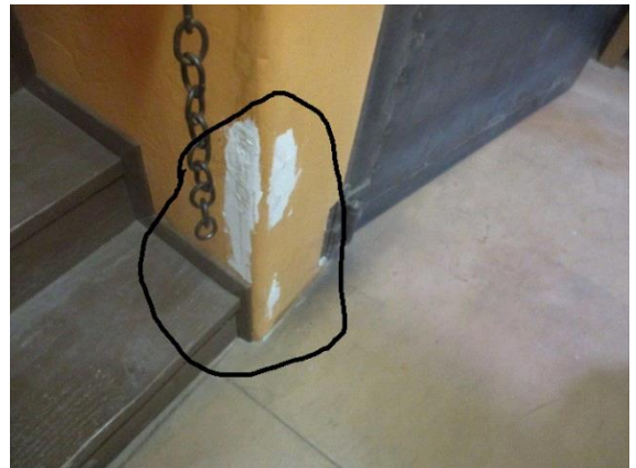
Stairs / Railings: Needs Paint
