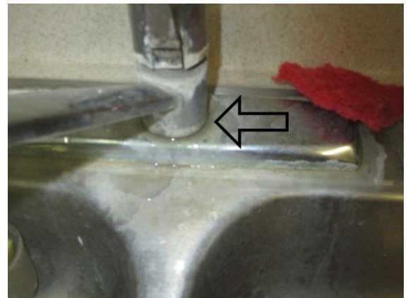
Break Room: Leak
