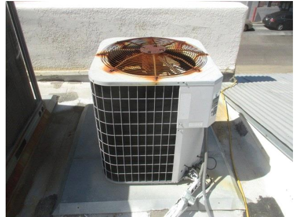
Cooling 2nd Floor :
