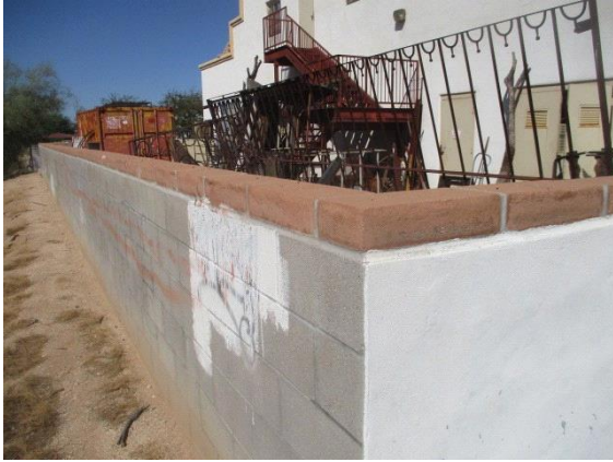
Fences / Enclosures: Graffiti
