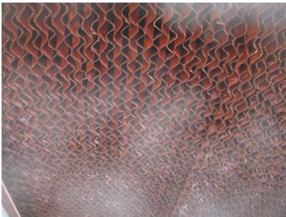
Cooling 1st Floor Rear:
