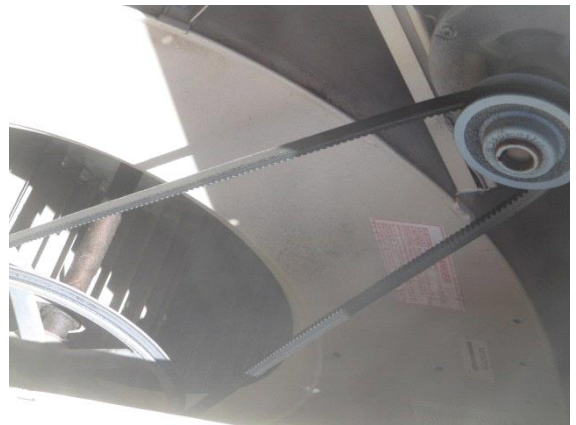
Cooling 1st Floor Rear:
