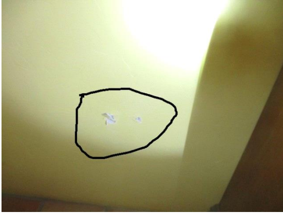
Upstairs Bathroom: Scratched Wall
