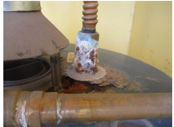
Water Heater: Deterioration
