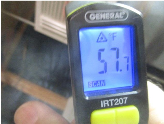
Cooling 2nd Floor :
