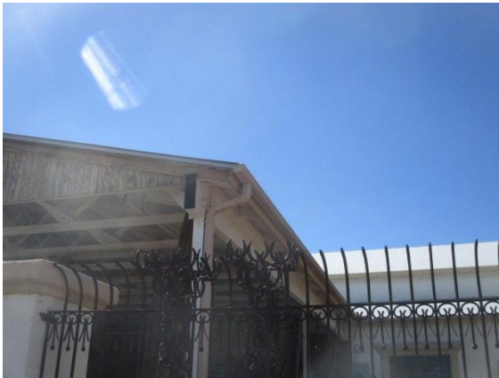
Roof Drainage System:
