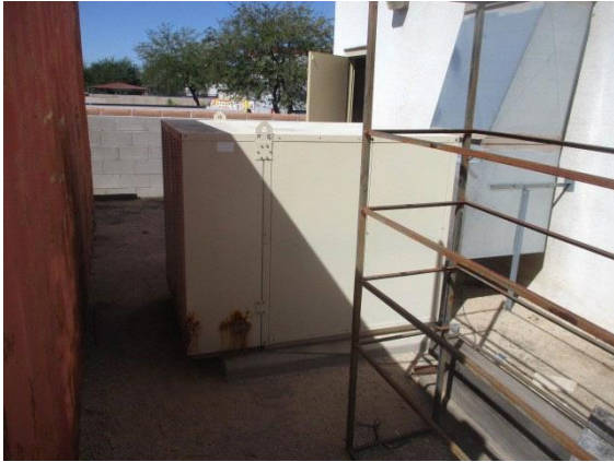
Cooling 1st Floor Rear:
