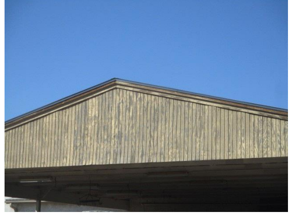
Covered Area: Needs Paint
