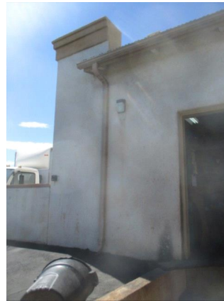
Roof Drainage System:
