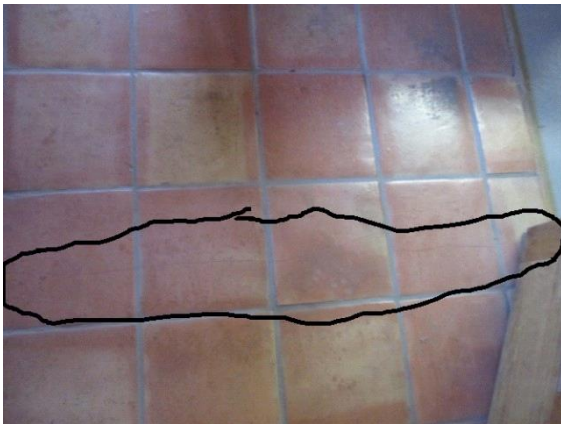
2nd Floor Storage & Office: Cracked Floor Tiles
