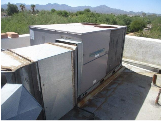
Cooling 1st Floor West:
