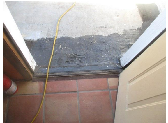
Roofing: Roof Leak At Door
